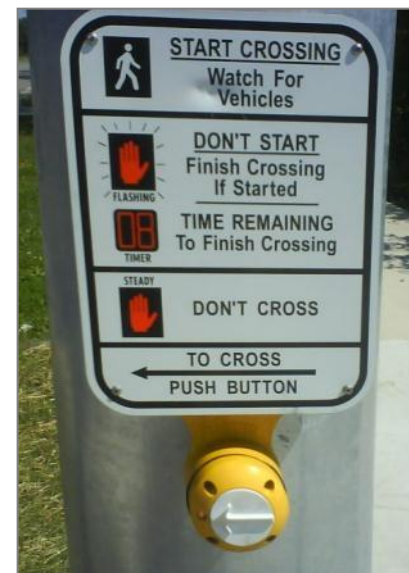
Figure 1: Photo of APS Installation
