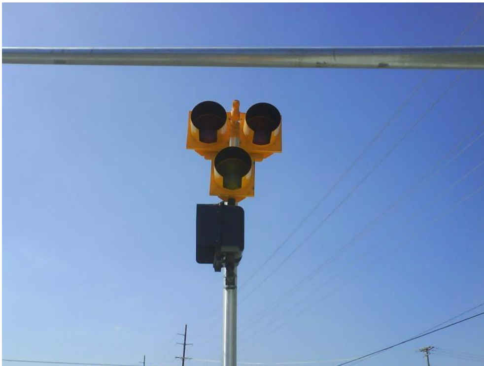
Figure 43: Close-up View of PHB at Maple at Drake Roundabout
